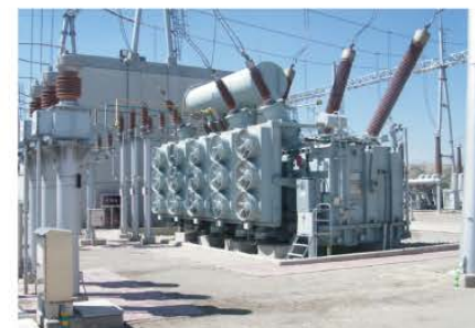
OSFPSZ-360000/330 transformer, operated at JISCO Yuzhong Iron & Steel Co., Ltd
