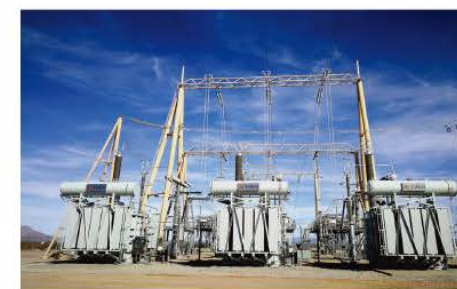
BKD-70000/525, BKD-58300/525 Reactor, operated at the project site of LADWP
