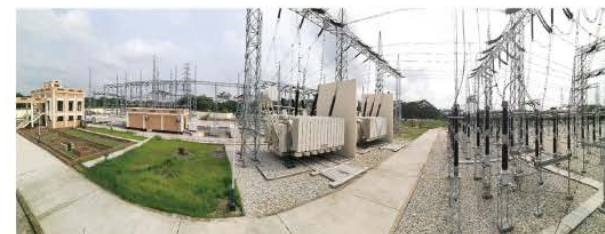
OSFZ-300000/230 transformer, operated at Barisal Substation in Bangladesh
