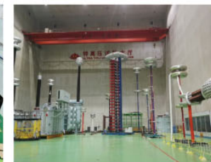
UHV test hall with a net height of 43 meters, CNAS certification, 1000kV and 1000kVA power transformer test base
