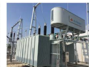
QYS-(16000+12500)/110 Railway traction transformer, operated at Zunyi urban section of Sichuan-Guizhou Railway
