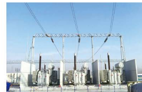
ODFS-334000/500 transformer, operated at Gaotang Substation in Liaocheng City, Shandong Province.
