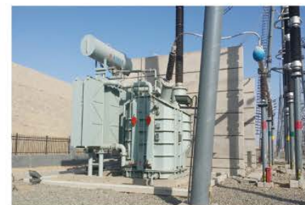
BKD-40000/500 reactor, operated at Xinjiang Hami Power Plant
